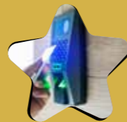
Access control entry
